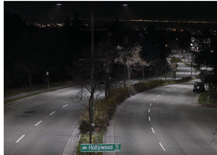
Above Right: GE Evolve installed in Oakland, CA. Image: http://www.businesswire.com/news/home/20140508006463/en/GE%E2%80%99s-LED-Street-Lighting-Installation-Demonstrates-Ongoing
