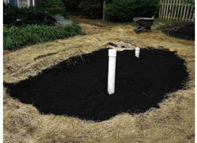
Straw covers the berm and soil around a recently built rain garden. The white PVC pipes allow for inspection of the underdrain and are not part of most home gardens.
