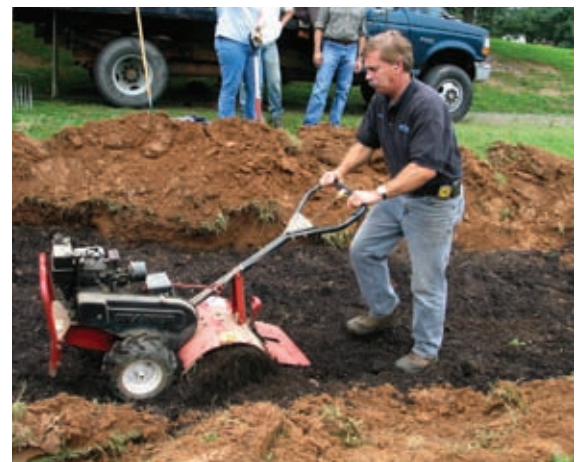
A rototiller is used to incorporate compost into the soil of a large rain garden in McLean.
