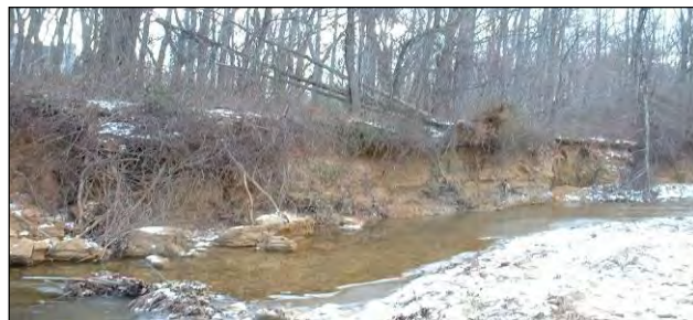
Severe erosion was observed at Scotts Run north of Old Dominion Drive
