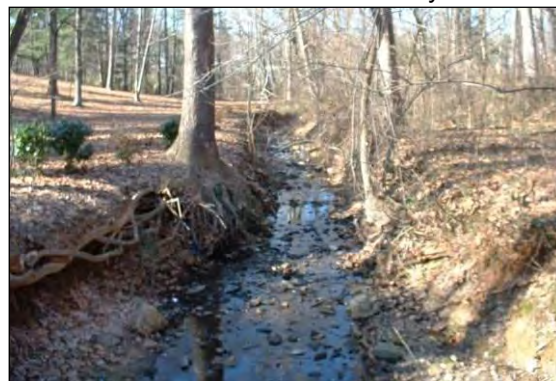
Eroded stream banks at a tributary to Dead Run near Churchill Road
