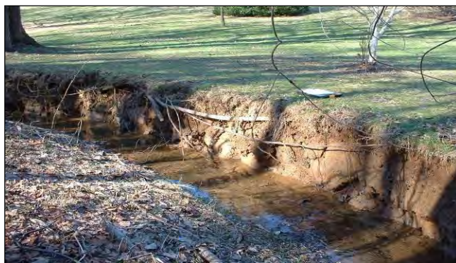
Severe erosion downstream of the Alvord Street crossing
