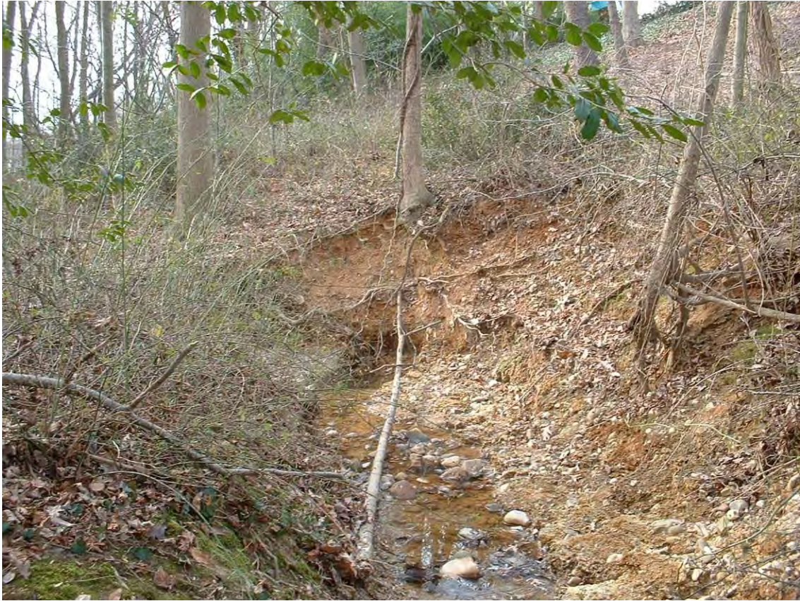
DC9201_1.jpg: Erosion on outside meander bend
