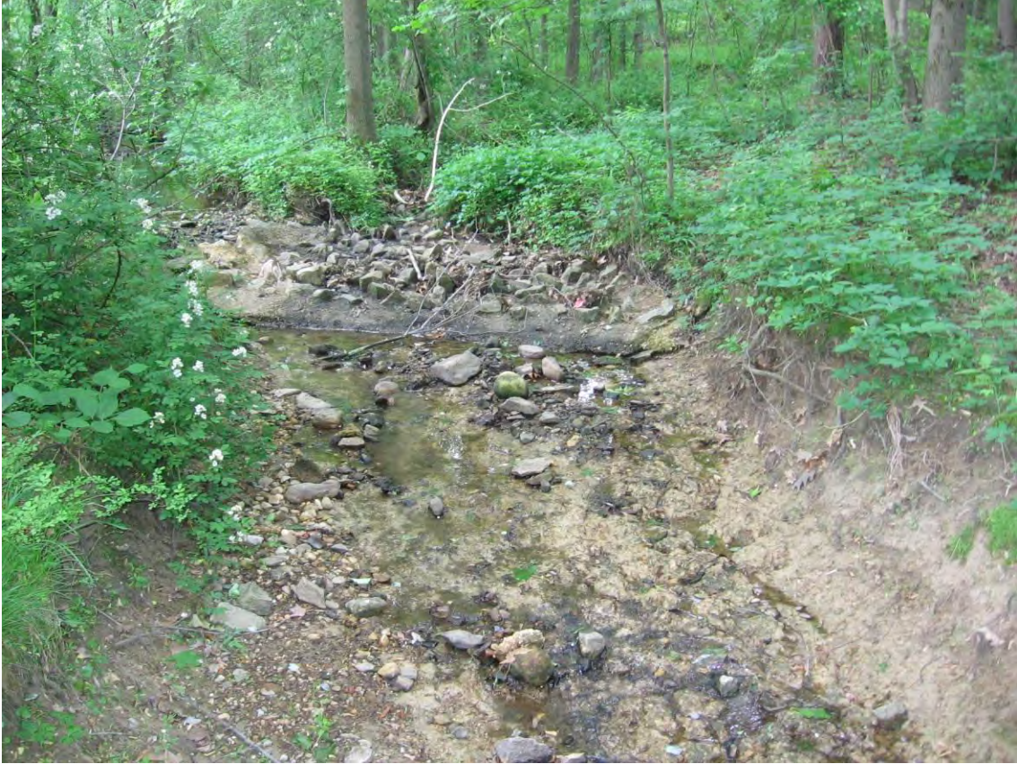
DC9204_1.jpg: Eroded and incised channel
