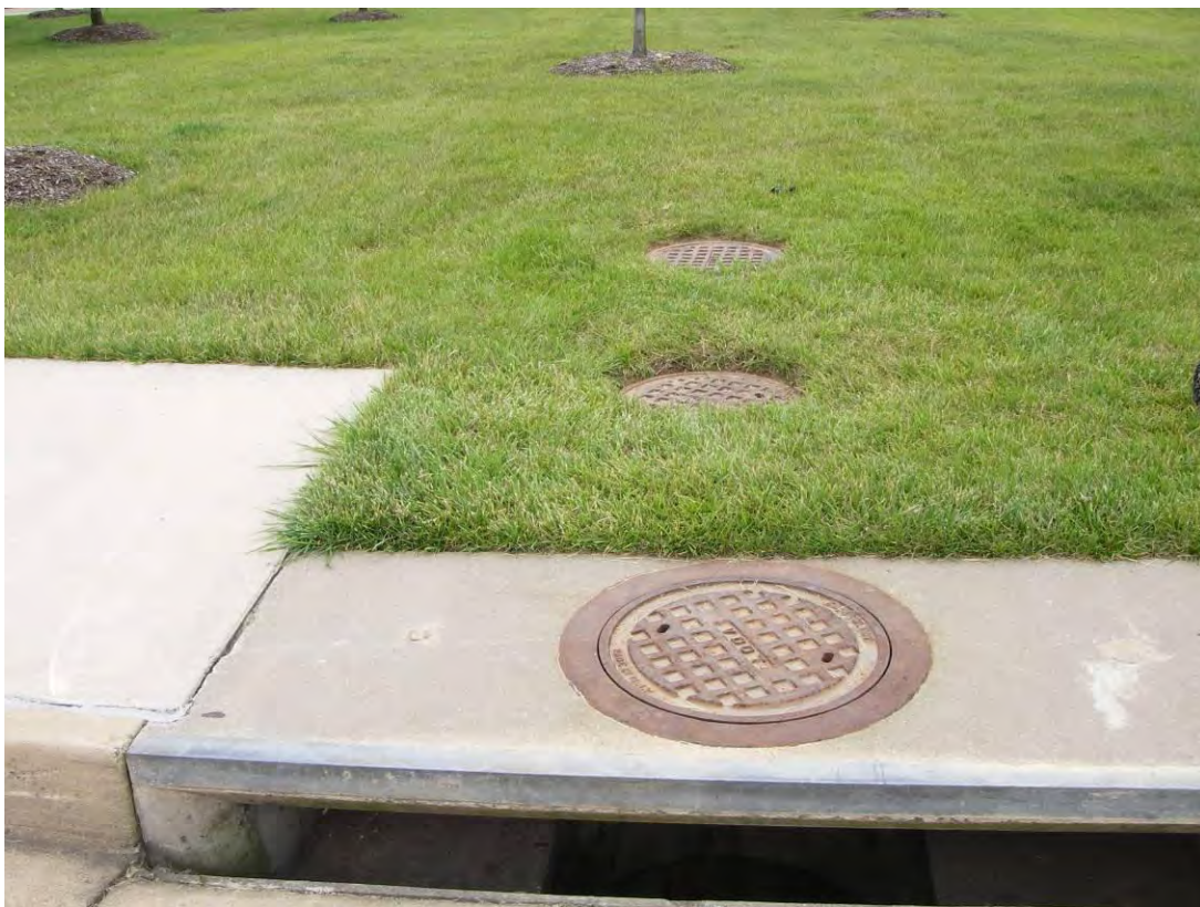
DC9518_2.jpg: Existing inlet in parking lot
