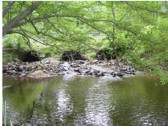
Figure 4-16: Obsolete culvert (Source: KCI)
