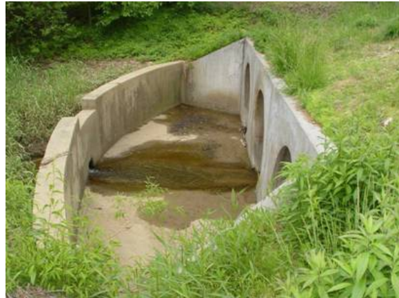
Figure 4-6: Culvert retrofit control structure, flow left to right (Source: KCI)
