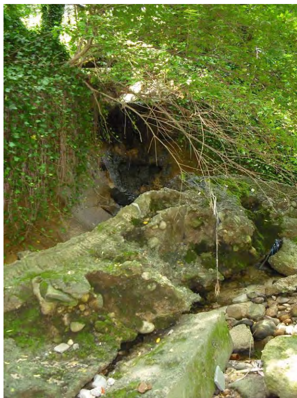
BE9200_2.jpg: View of erosion along the banks
