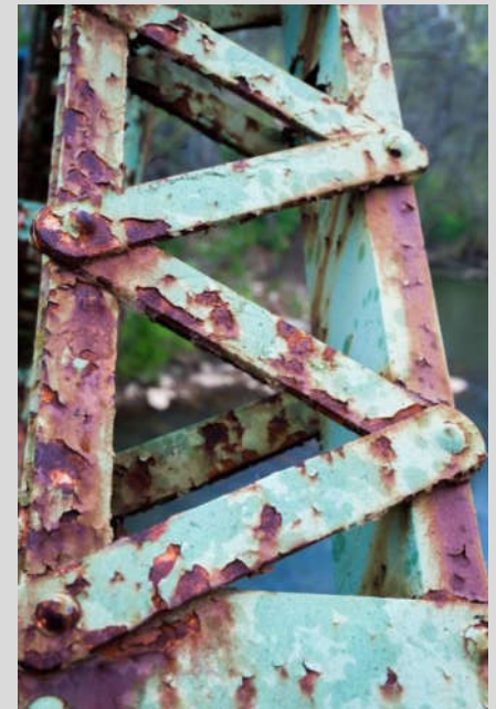
Bridge corrosion Photo by Jim Palmer.
